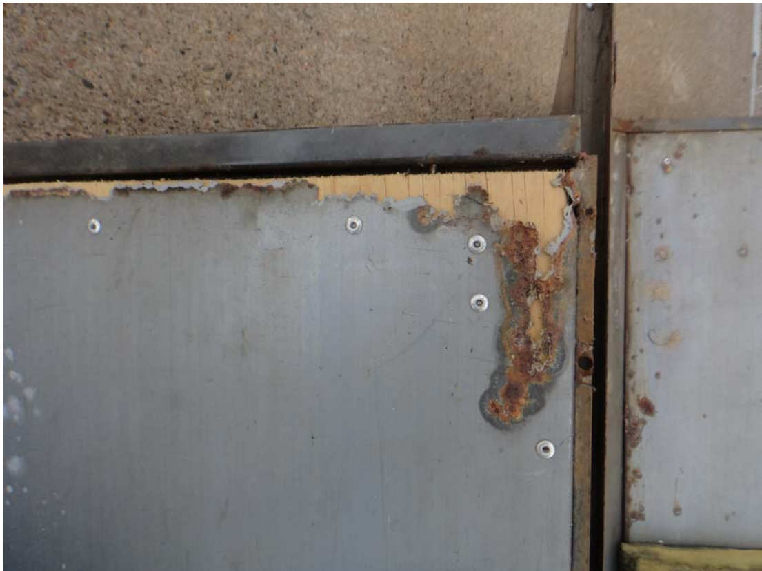
Photo 21 Corner Deterioration at Back of Panel.JPG
