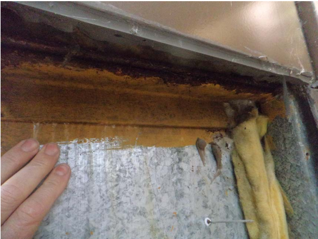
Photo 11 Close up at Top of Removed Panel.JPG
