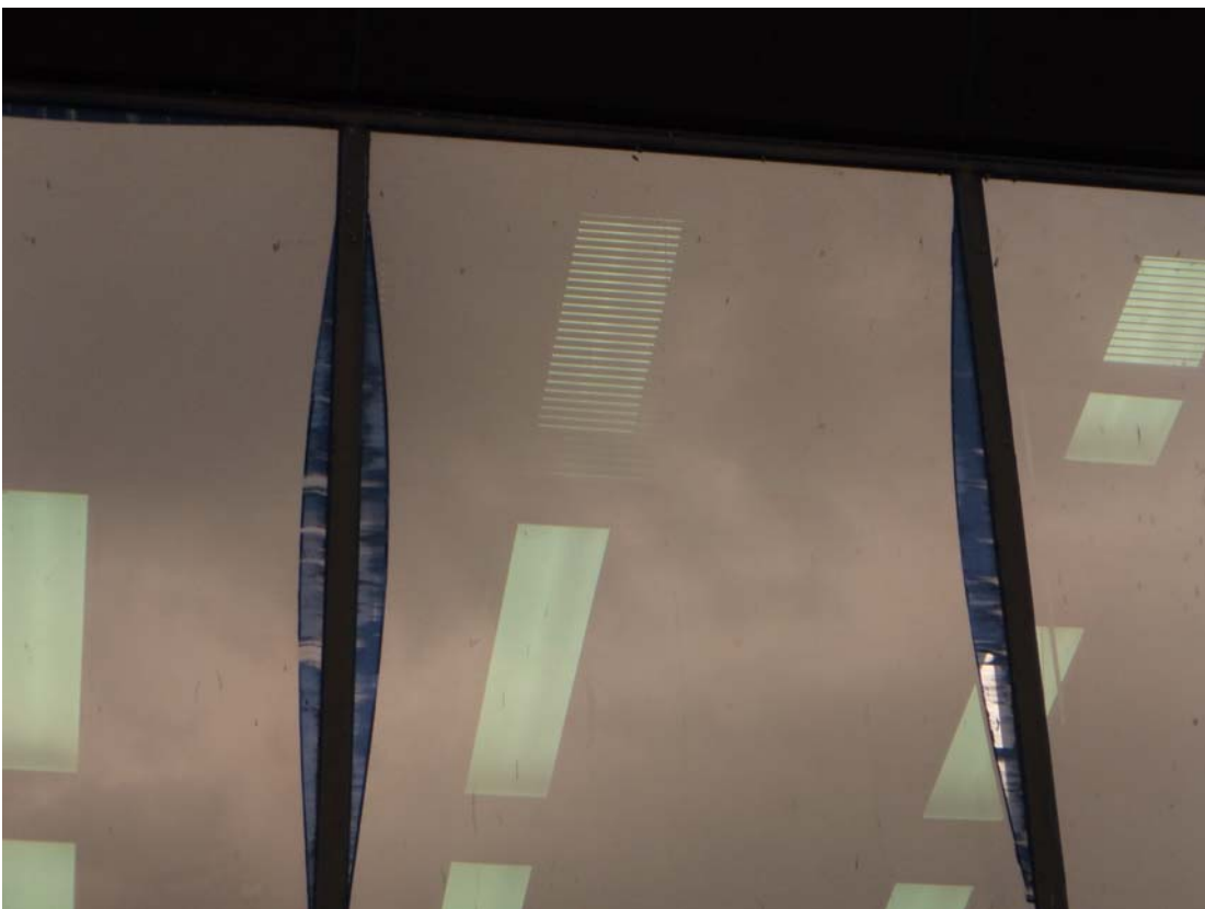
Photo 26 Window with Failed Spacer.JPG
